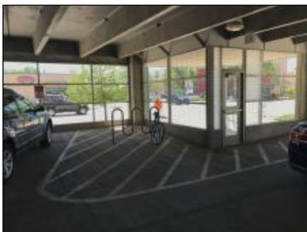
Finding 297249 Additional Photo
