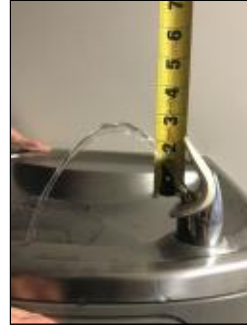
Finding 299188 Additional Photo
